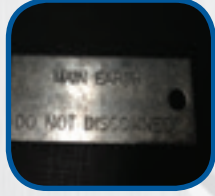
Earth Rods Safety Tag
