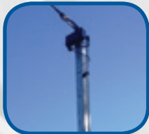
Mains Supply Support Pole
