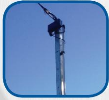
Mains Supply Support Pole
