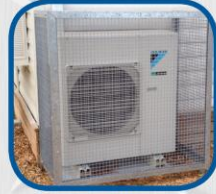
Air Conditioning Condenser Cage
