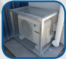
Air Conditioning Condenser Cage
