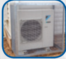
Air Conditioning Condenser Cage
