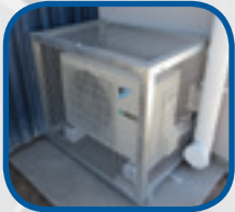
Air Conditioning Condenser Cage
